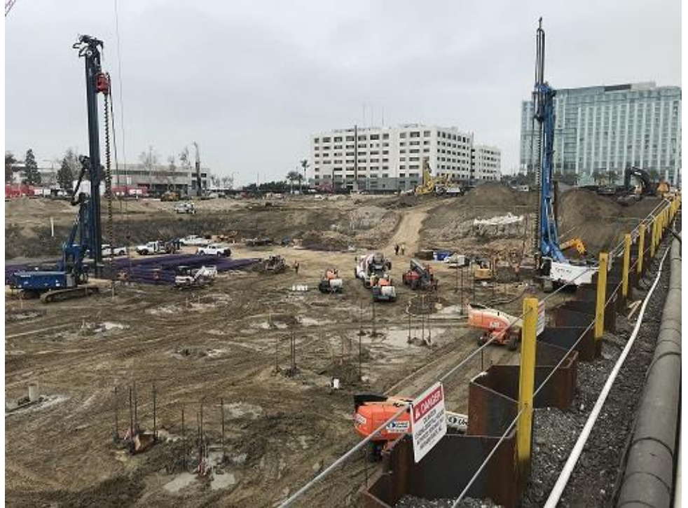
Sheet Piles and Auger Piles for Pacific Gateway in San Diego, California.
